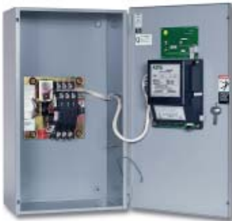
Fig. 2: ASCO Power Transfer Switch rated 200 amperes
