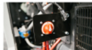
Battery Shut-off Switch
