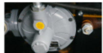
Installed Gas Regulator
