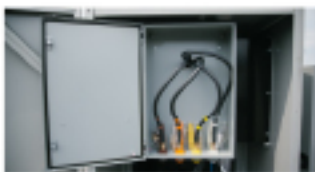
Power Distribution Box with Camlocks
